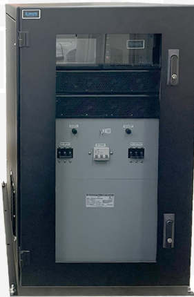
NEDM Three-Phase 20 kVA UPS with Galvanic Isolation Transformer (est. 251 Lbs.)
