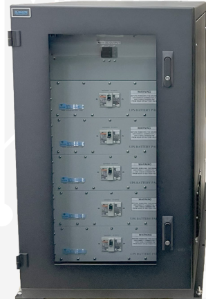
Battery Cabinet with 5 VRLA Battery Drawers and Protective Circuit Breakers (est. 944 Lbs.)
