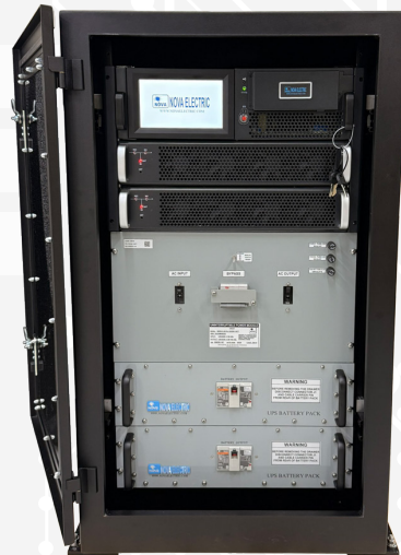
20 KVA THREE PHASE UPS WITH 2 BATTERY DRAWERS AND I/O CIRCUIT BREAKER PANEL
